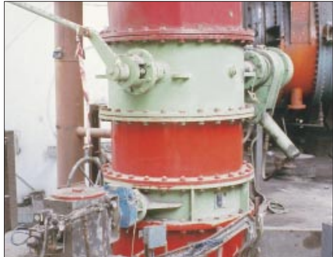
▲ Gas Safety Shut-off Valve (Three-Lever Valve, top) and Gas Flow Control Valve (Clearance-type Butterfly Valve, bottom) in 1100 mm Stove Area Gas Line
