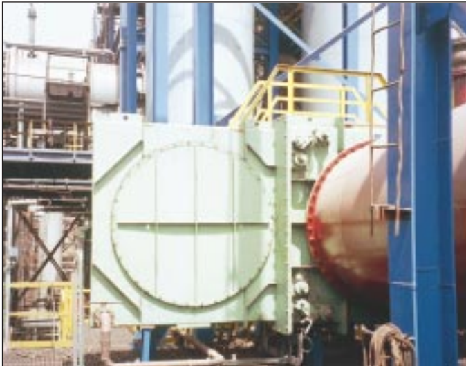
▲ 2000 mm Goggle Valve installed in clean gas line in Gas Cleaning Plant
